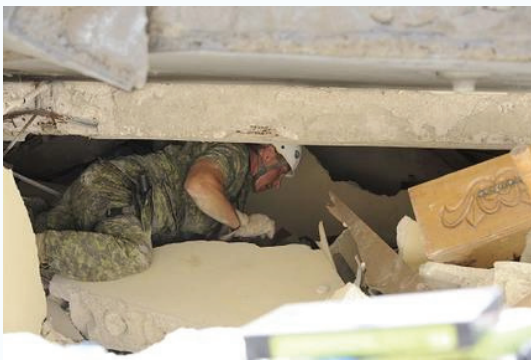
Captain Dez Desjardins, Urban Search and Rescue (USAR), searches for a missing Canadian in the ruins of a house in Port-au-Prince, Haiti.
